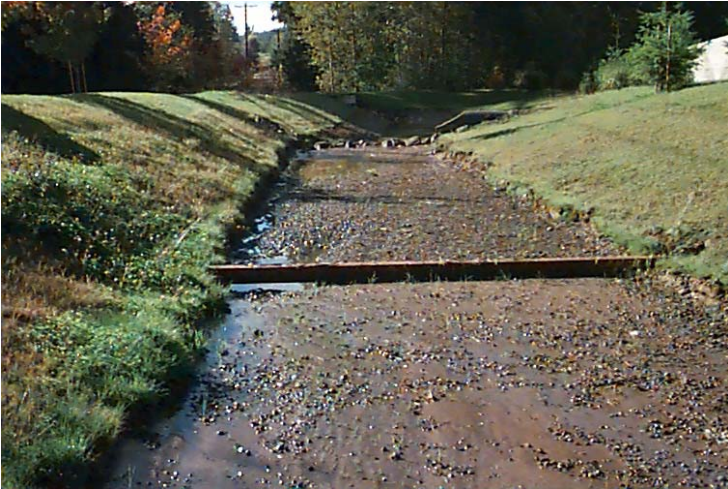
Within one year of construction
